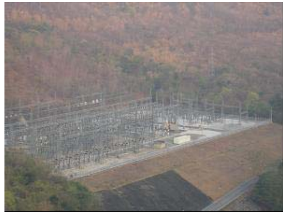
Switch Yard facility for distribution of power
