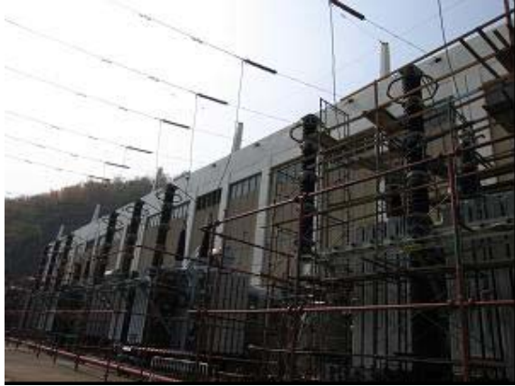
Transformer facility at Srinakharin Dam (37 KV transmission)
